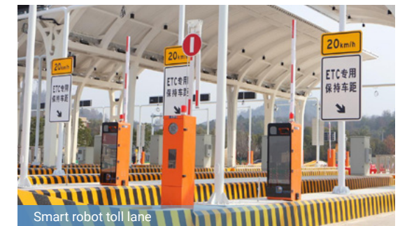
Smart robot toll lane
